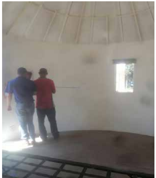
The EPWP beneficiaries at the Koekenaap cultural facility conducted repairs to the walls of the rondawel, after flood damage.
